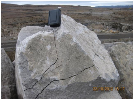
Figure 6. Fractured riprap stone.
