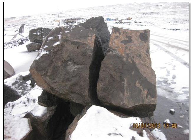
Figure 10. Another fractured riprap stone in the site test
