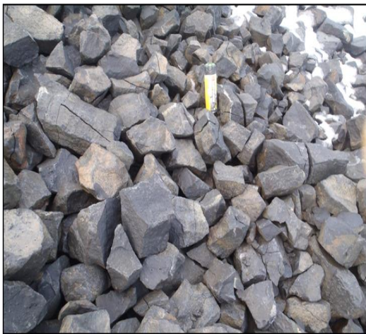
Figure 14. Frost fractured slope protection materials in autumn 2012.
