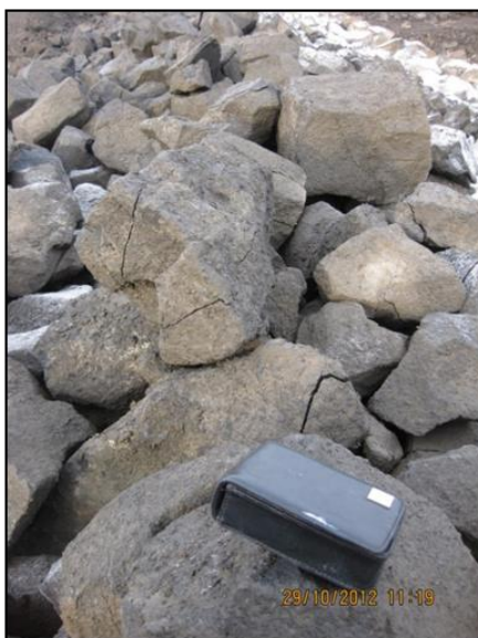
Figure 15. Frost fractured slope protection materials in autumn 2012.
